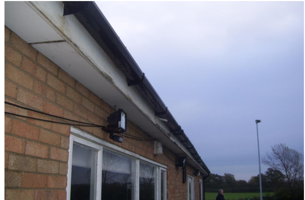
Fascias, Soffits & Gutters Require Maintenance
