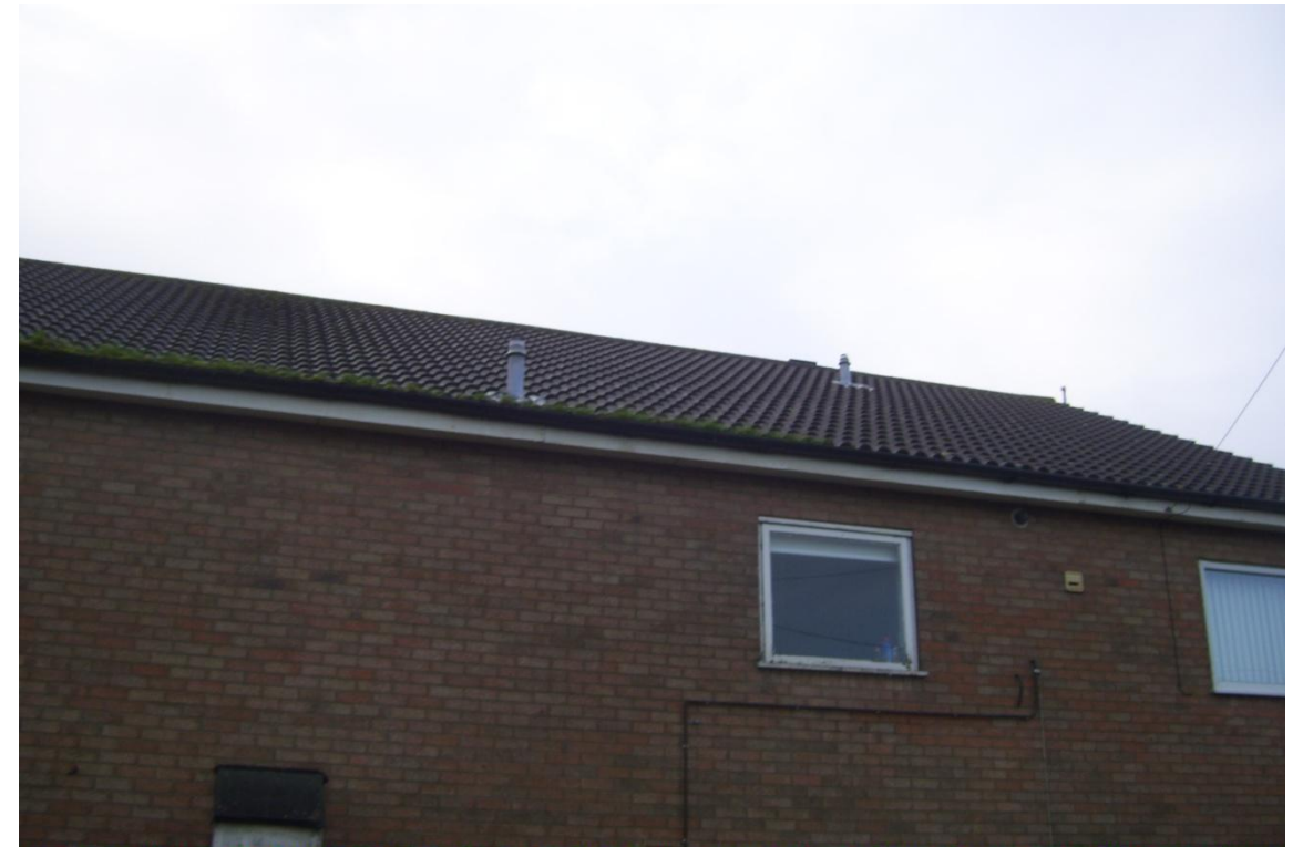
Gutters are clogged, roof tiles in good condition and single glazed windows.
