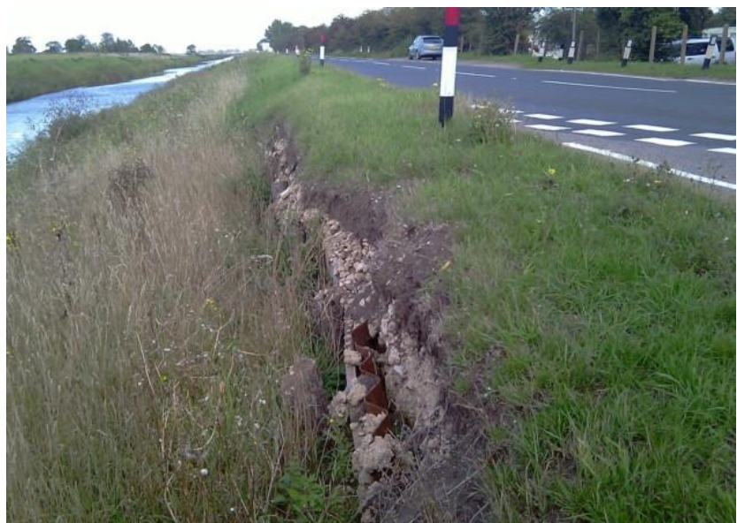
Embankment slipping at Sixteen Foot Bank near Stonea in Fenland
