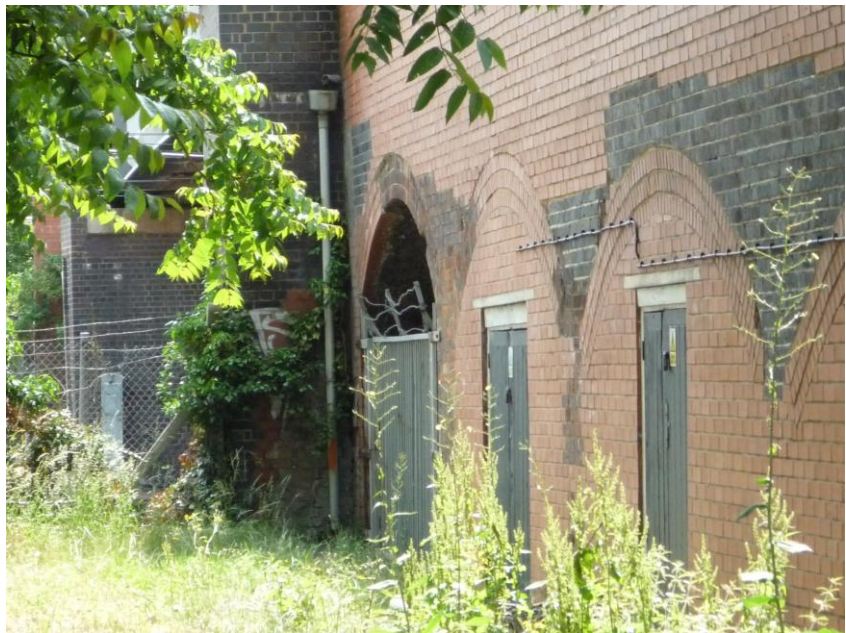
Arch of the Mill Road bridge under which it is planned to take the Chisholm Trail into the Cambridge Station area.
