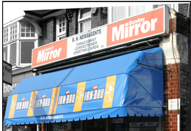
Inappropriate Dutch style canopy with over-dominant advertising
