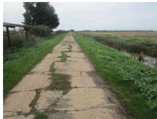
Figure 7A.10.2 The poor surfacing presumably extends from the edge of the public highway at Maedlands Farm to Cran Brook, but has not been surveyed. (View towards gate from near Maedlands Farm.).
