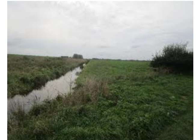
Figure 7A.7.7 View along flood bank towards Sutton showing the public footpath as almost impassable.
