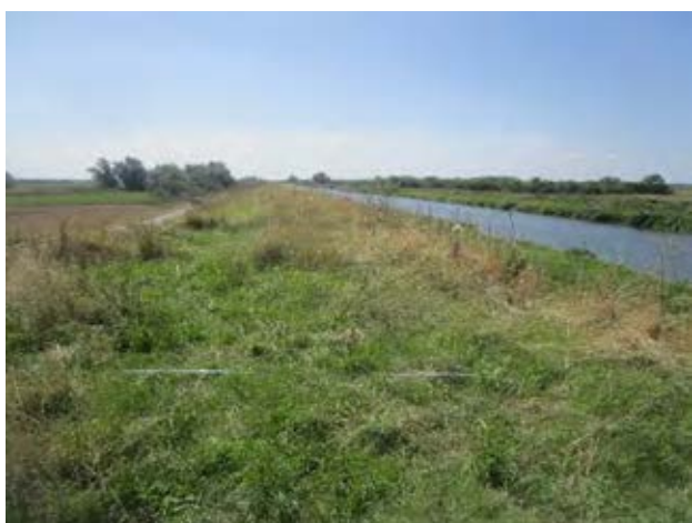
Figure 7D 5.1 View of the bank top with 3m tape just visible. Looking towards Earith. The bank is only just over 3m wide so any edge detail would be very difficult for a 3m path.
