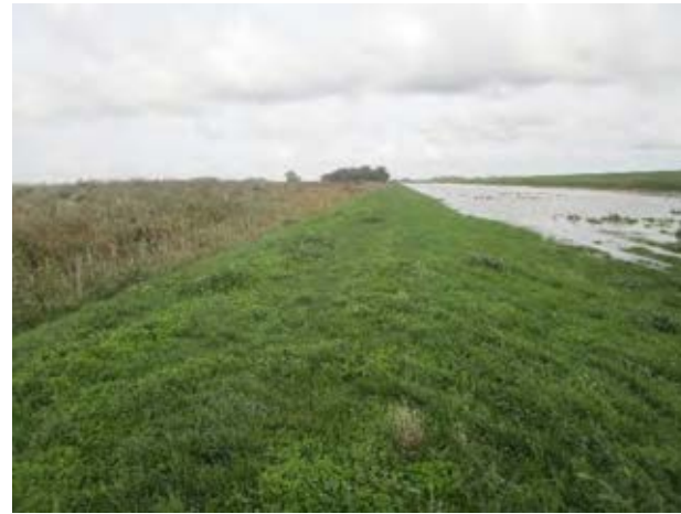
Figure 7A.7.1 View along flood bank towards Sutton with flooded field to right and watercourse to left.
