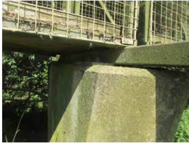
Figure 7A.16.8. The existing support arrangement. Detailed design is needed to see if it can be retained with a new bridge arrangement as adjacent.
