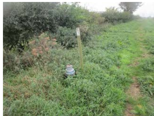
Figure 7A.10.2 Valve assumed to be for water supply adjacent to field edge path.
