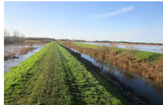
Figure 7C8.3 Eastern banktop, Lode and fields in winter. The suggested path would be in the fields on the right. View towards Cottenham.
