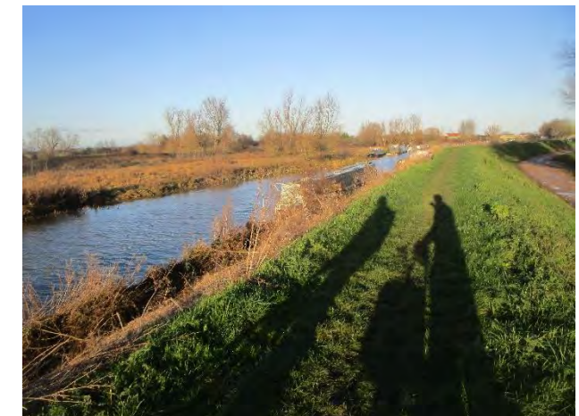
Figure 7F10.3 View along south bank showing narrow bank top. The access road adjacent is not continuous and is in poor condition. The existing river bridge is not suitable for all.
