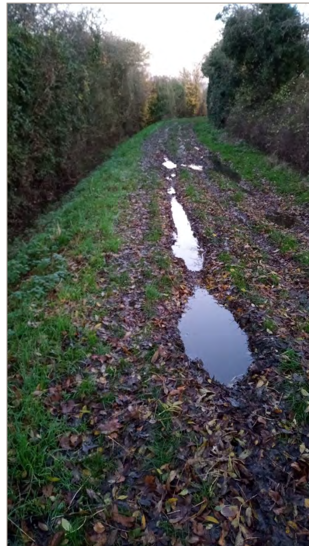
Figure 7B11.1 View of public byway. It is in variable condition and will need detailed surveys and major works.
