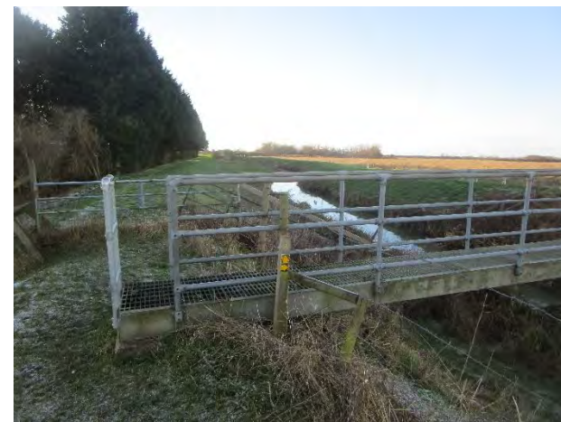
Figure 7C9.3 The existing bridge over Cottenham Lode. A wider bridge would be needed for the route in a similar location.
