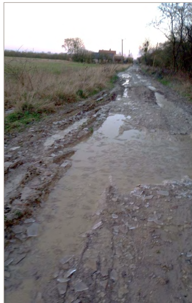
Figure 7E4.2 Church Lane is in very poor condition in places.
