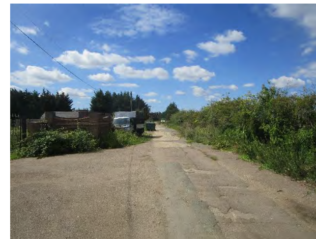
Figure 7B4.1 Lockspit Hall Drove at Setchel Drove junction showing the poor surface.
