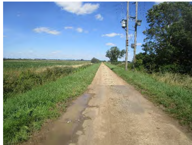
Figure 7A6.1 Lockspit Hall Drove – a full survey would be needed to determine the extent of works needed to provide a smooth, durable surface.
