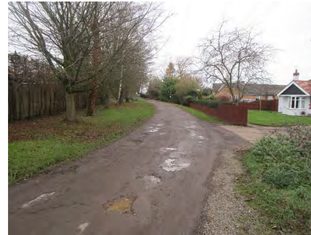
Figure 7A.19.1 Hinton Way, Wilburton needs resurfacing.
