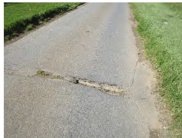
Figure 7E5.2 Long Drove showing an extreme example of cracking.
