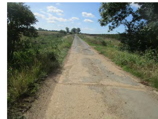
Figure 7E6.2 The uncomfortable nature of the surfacing is evident.
