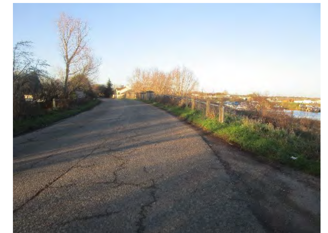
Figure 7F9.1 View along former A10 with Marina and the bridge over the River Great Ouse visible.
