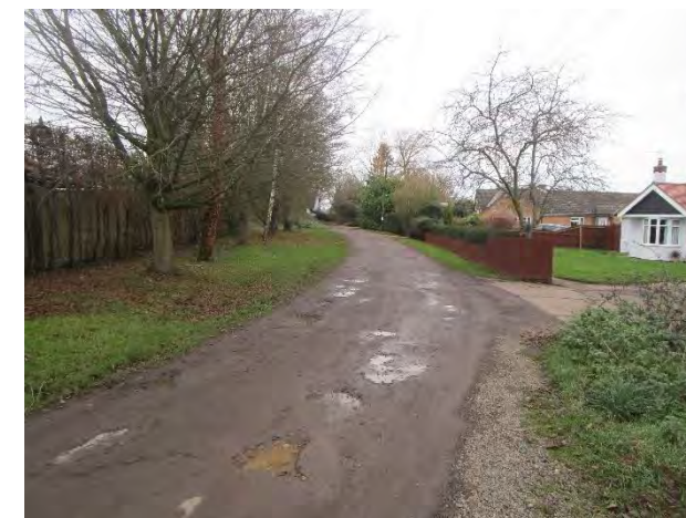
Figure 7B.15.1 Hinton Way, Wilburton needs resurfacing.
