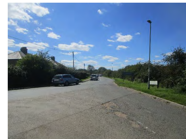
Figure 7A4.1 Smithy Lane view towards 7A3.2 and Cottenham, showing surface issues on Smithy Lane and difficulties at the junction that need addressing.
